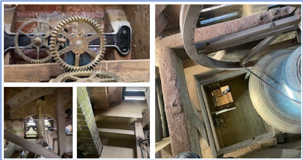
Photos of the clock installation – the new platform features in the bottom centre photo
